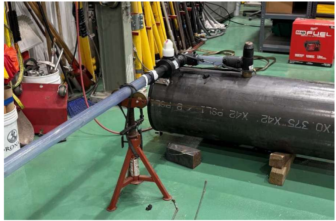
Service line configuration including 2-in PE piping, elbow and ball valve.
