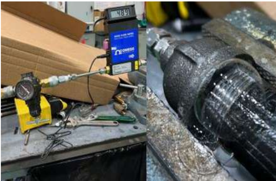
Flow rate of the leak.
