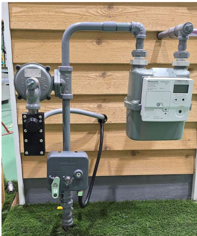
Prototype testing setup for evaluating service regulator and meter performance
