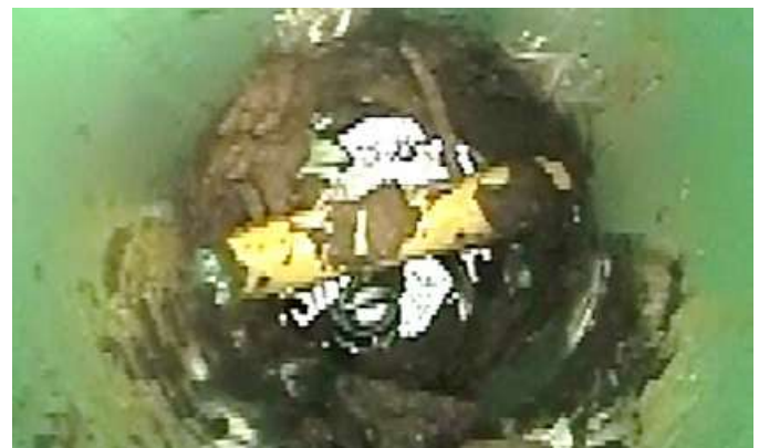
Blockage caused by Cross-Bore in Sewer Line
