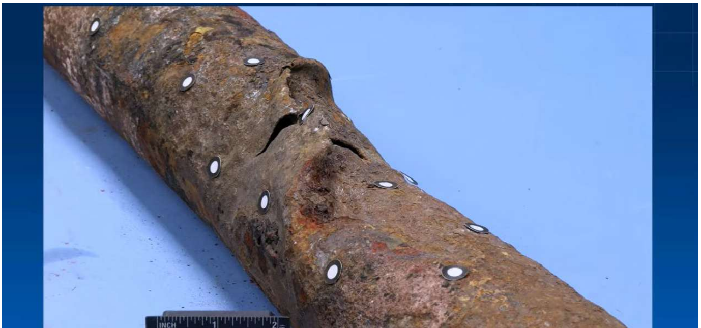
Steam Pipe External Corrosion, Buckling, and Cracking
